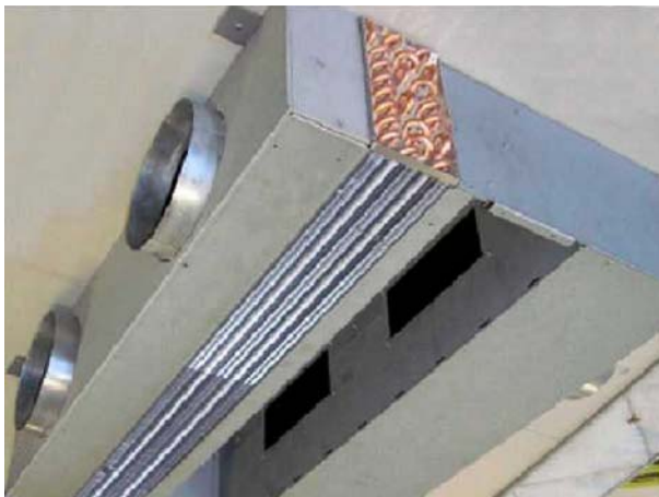
3. Removal of lower plate / vacuum-cleaning of heat exchanger on the pressure side
